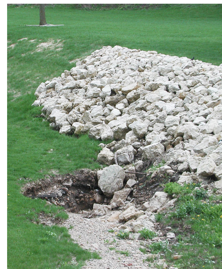
Sinkhole, rapid development —Unconsolidated surficial deposits have collapsed into cavities developed in the underlying bedrock of the Prairie du Chien Group. This 2 meter wide sinkhole was first observed in 2001, and probably developed (or redeveloped) during heavy rain and snowmelt in the spring of that year. Rapid development of sinkholes in this manner is common in southeastern Minnesota. (Boulders of bedrock above the sinkhole are rip-rap used to hinder streambank erosion).
